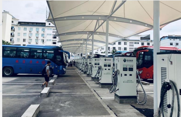
Shanxi State Grid Project
