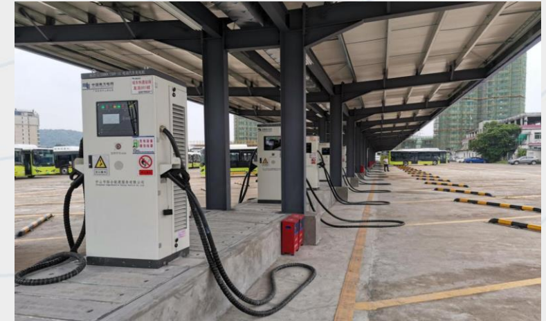
Tianjin State Grid Project
